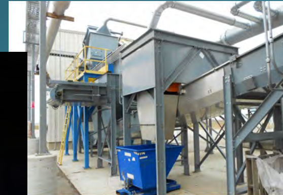
Sludge Drying and Pelletizing Plant - Chicago
